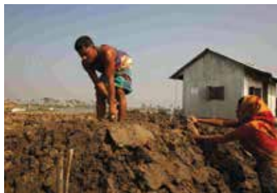
Instead of engaging in shrimp farming, which is degrading to the environment, Marufa in Kaligunj, Satkhira, Bangladesh, is constructing a plinth for his family's house, raising it above flood levels. Making a plinth is done by constructing ponds for rainwater harvesting, which are used for vegetable growing, an environmentally benign alternative to shrimp farming. Photo by Mahmud.
